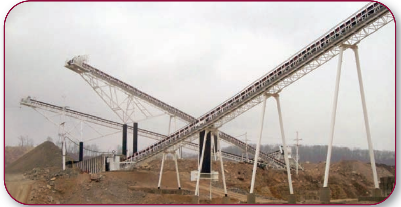
(2) 42" x 274" Stationary Surge Pile Conveyors 42" x 704' Tunnel Feed Conveyor (Front)
